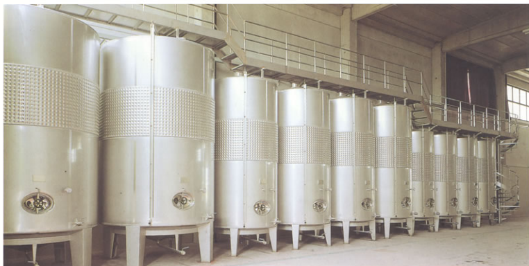
■ Thermo-conditionated storage tanks.
