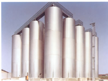
■ Flat-bottomed storage tanks.
